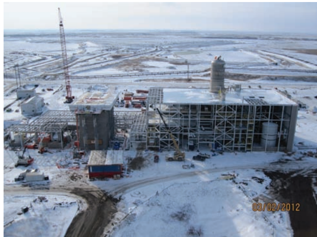
General view of the 1 Mt/year CO 2 capture plant under construction at the SaskPower Boundary Dam Generating Station near Estevan, Saskatchewan, Canada. (Courtesy: SaskPower)
